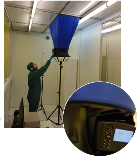
Facility Manager testing the airflow (blue funnel) and the noise.
